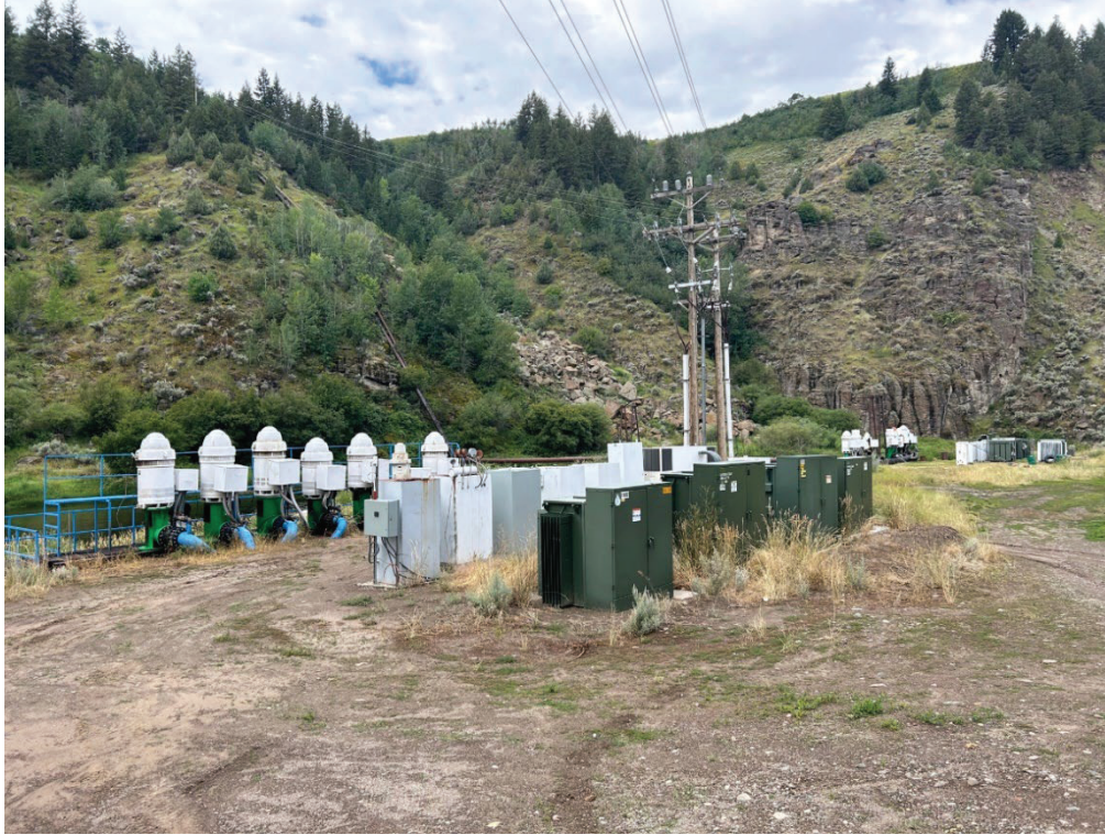
Figure 2. Schwendiman site pumpstation, situated in cleared vehicle access area at river left of the Teton River.
