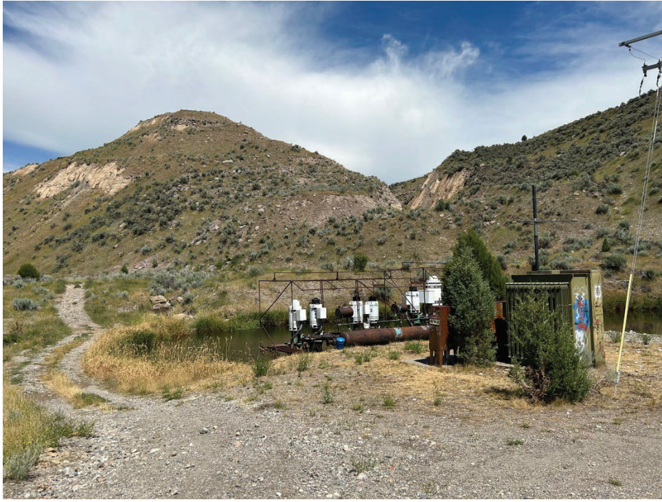
Figure 8. Canyon Creek Lateral POD pumpstation with part of Pond B visible at right, taken from downstream side (facing upstream). The Teton River is to the left out of photo frame. Access road leading to canyon rim visible at left.
